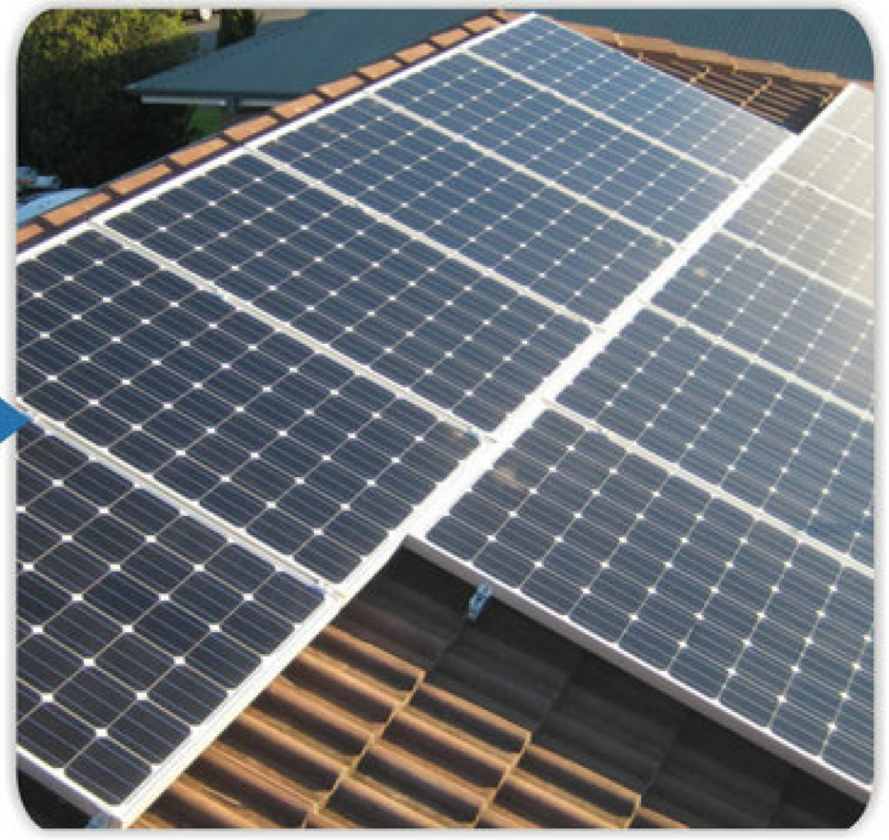
3kw tile roof
