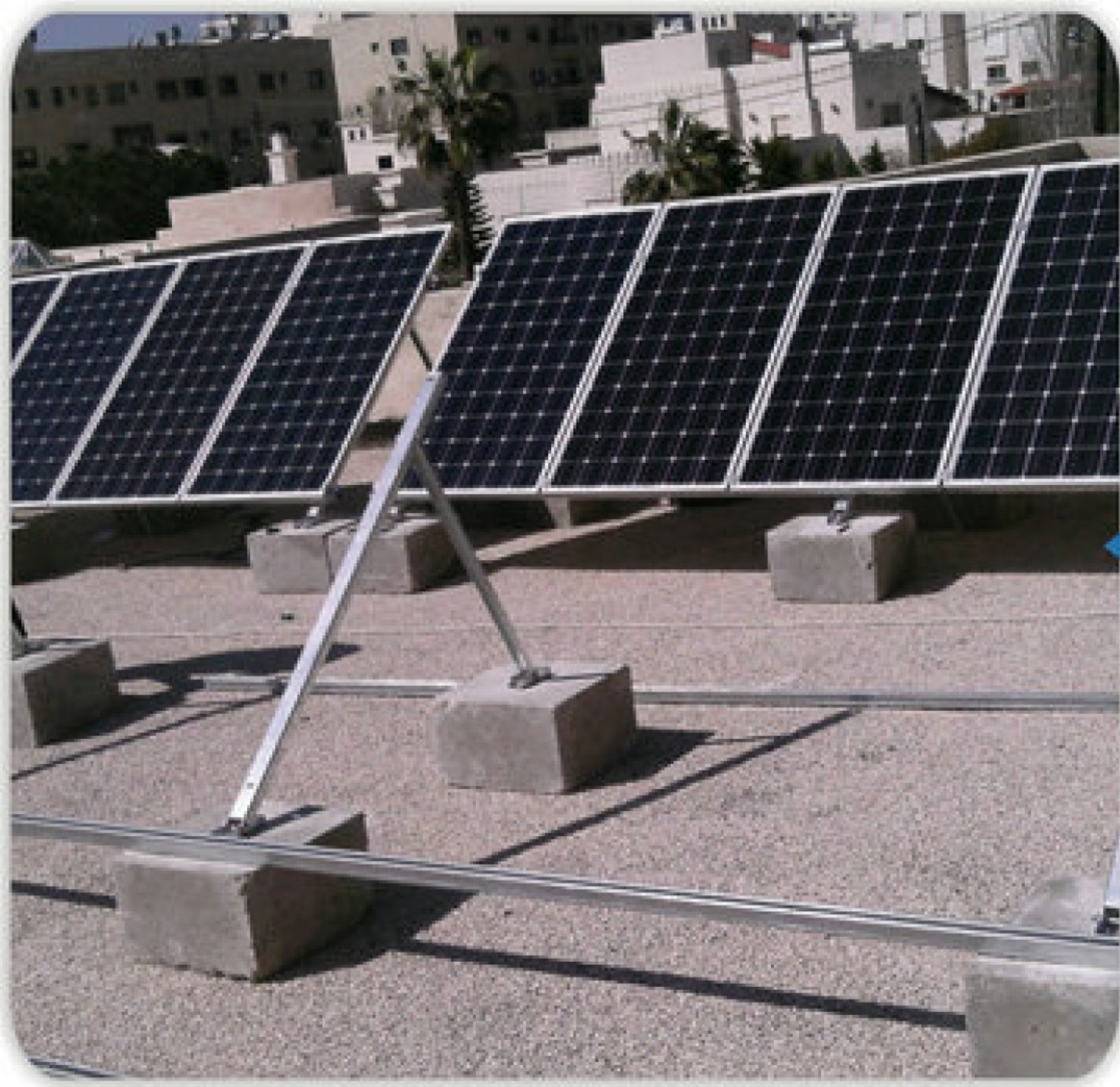
5kw flat roof
