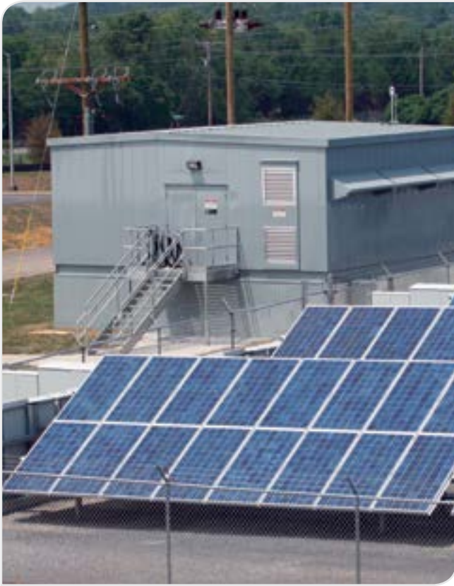
Tennessee, USA PV power plant 1 MW
