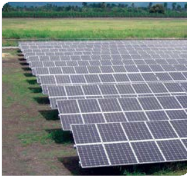
Cibao, Dominican Republic PV power plant 1.5 MW
