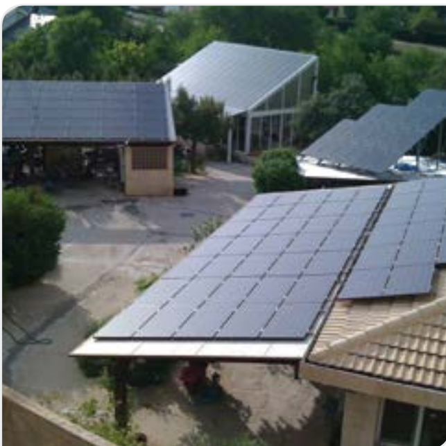
Madrid, Spain Off-grid solar 18 kW
