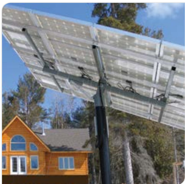
Ontario, Canada Off-grid solar 10 kW
