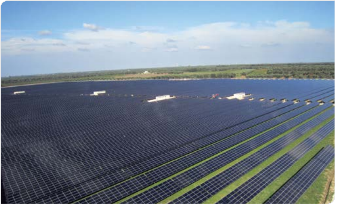
Puglia, Italy PV power plant 43 MW
