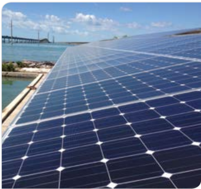
Florida, USA PV power plant 23 kW
